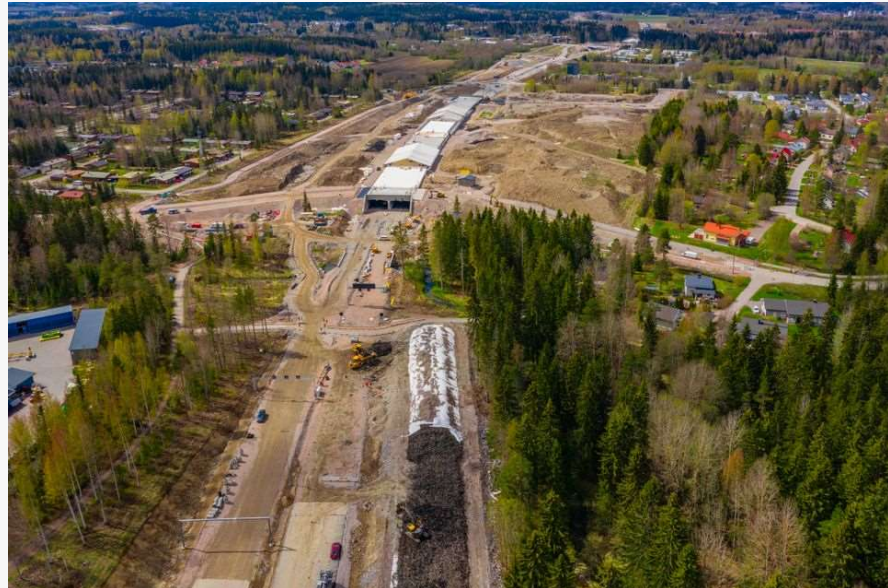
Picture: Skanska. The Patomäki tunnel under construction. The tunnel was decided to be shortened during the development phase, which reduced the project's emissions and the amount of technology used.
